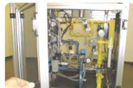
Hinged door provides easy access to utilities and heat controls.
